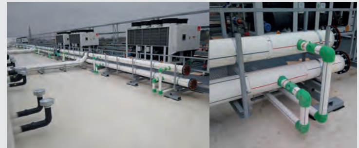
Data Center, Italy
