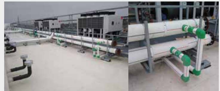
Data Center, Italy
